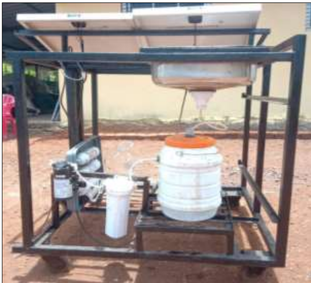
Fig 2: Developed solar PV powered brackish water desalination unit
