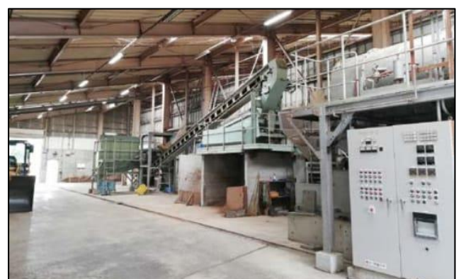
Fig 8: Mechanical separation after fermentation process
